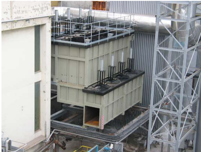
Abb. 5: MVA Paris, Carrier-sur-Seine [Quelle: Shell, environmental catalysts & systems].
